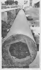
Looking down the barrel of a cannon! Here are several sections of the "Big Inch" lying on the ground near the paint shop. 4000 feet of this big pipe will be installed this month.
